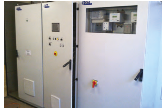
The excitation equipment manufactured by ČKD was commissioned in September 2013.
