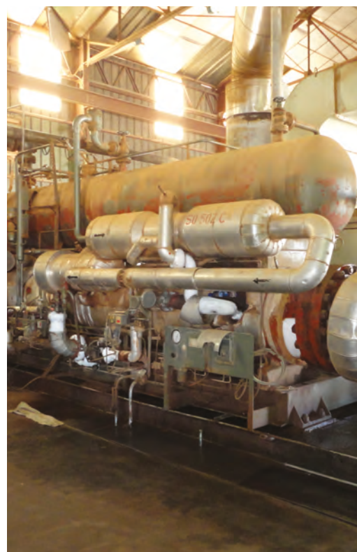
The previous technological system, which will be replaced with a new cooling unit located in a new hall
